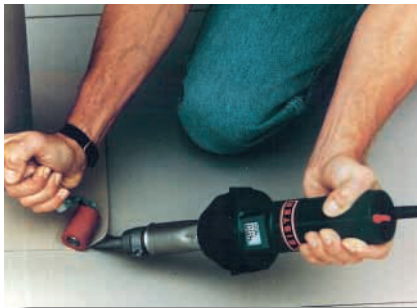
TRIAC PID with 20 mm wide slot nozzle and pressure roller being used to weld TPO roofing membranes.
