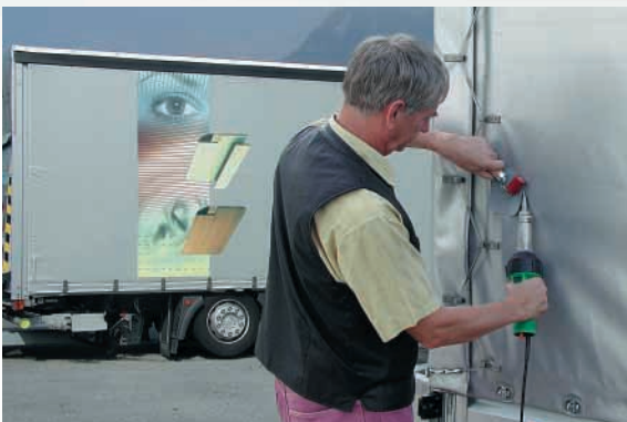
TRIAC PID with 20 mm wide slot nozzle and pressure roller being used for repair welding on a tarpaulin.
